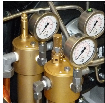
Safety valve 1st and 2nd stage
