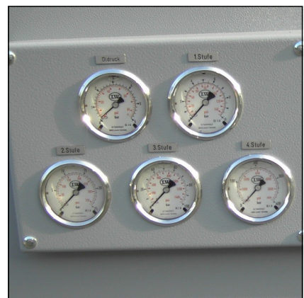
Fig. 2 - Interstage pressure gauges in SILENT HOUSING
