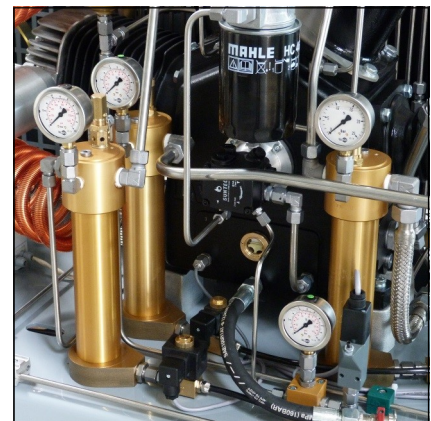
Oil / water separators 1st, 2nd and 3rd stage
