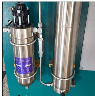
Fig. 3 - Loose pipe connections and nuts
