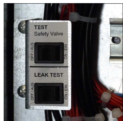
Safety valve test switch (up)
