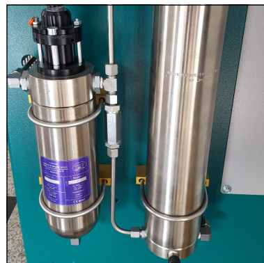
Fig. 3 - Loose pipe connections and nuts
