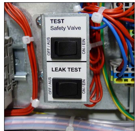
Safety Valve Test Switch (up)
