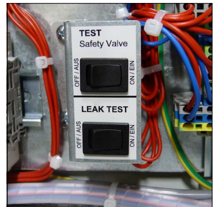
Leak test switch (lower)
