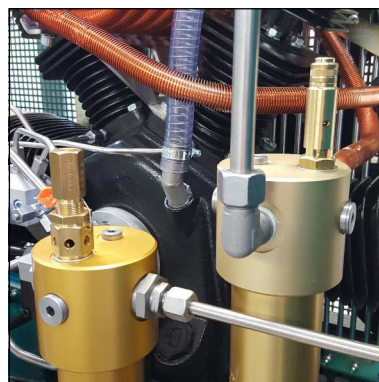
Safety valve 2nd and 3rd stage
