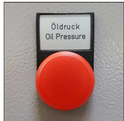
Oil Pressure Monitoring
