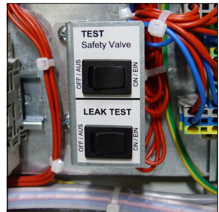
Leak test switch (lower)
