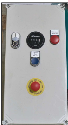
Condensate Test Drain Button
