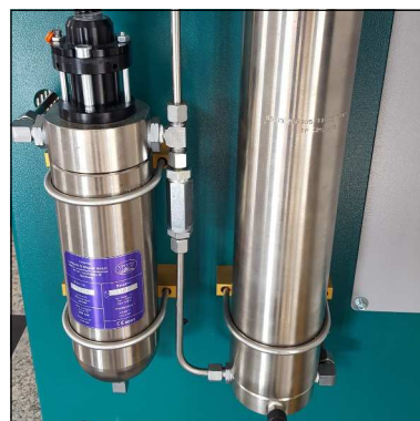
Fig. 3 - Loose pipe connections and nuts
