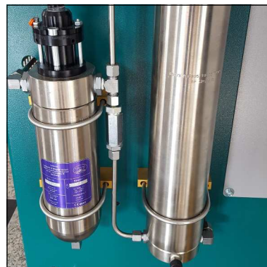
Fig. 3 - Loose pipe connections and nuts
