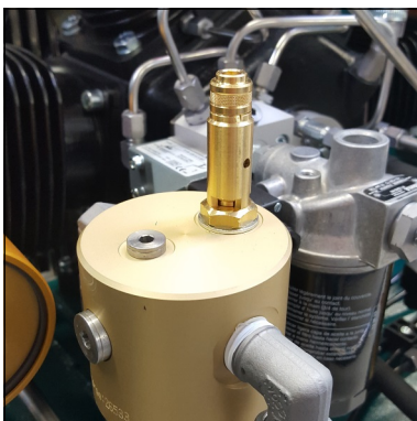
Safety valve 1st stage
