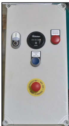
Condensate Test Drain Button
