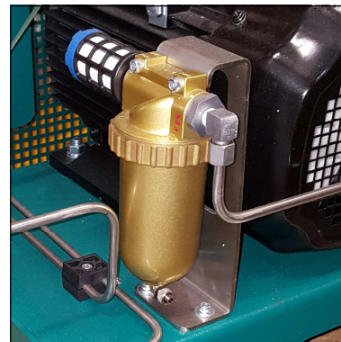
Oil / water separators final stage
