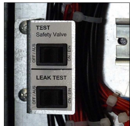
Leak test switch (lower)
