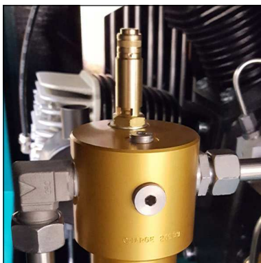
Safety valve 1st stage
