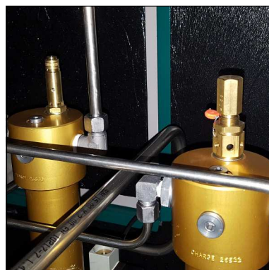
Safety valve 2nd and 3rd stage
