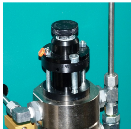
Safety valve 3rd stage
