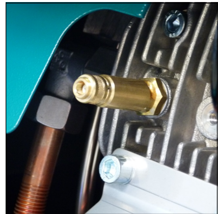
Safety valve 1st stage
