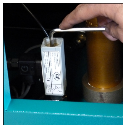
Final pressure switch
