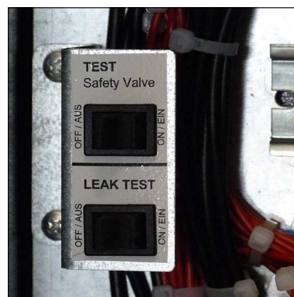
Safety valve test switch (up)
