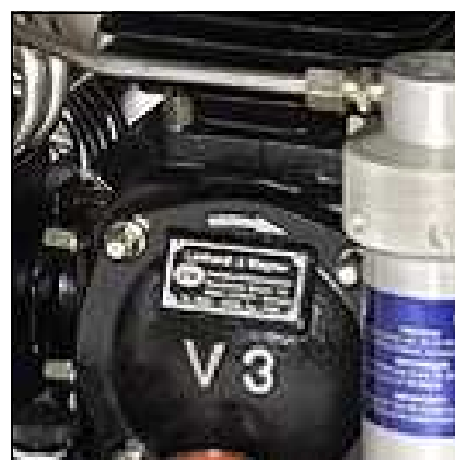
Rotation direction arrow on the compressor block
