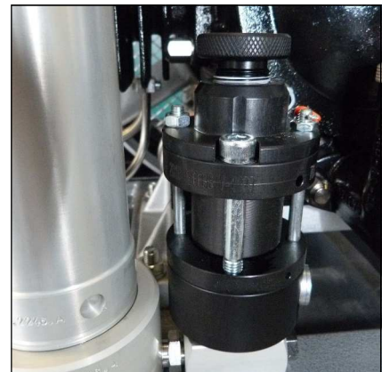
Fig. 2 - Safety valve 3rd stage
