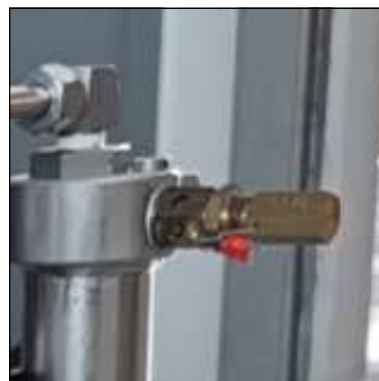
Safety valve 2nd stage
