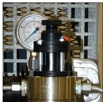
Safety valve 4th stage
