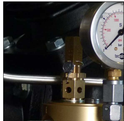
Safety valve 3rd stage
