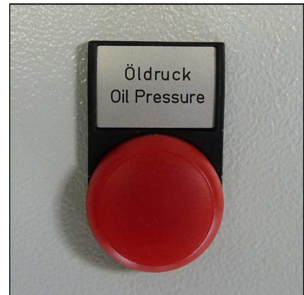
Oil Pressure Monitoring
