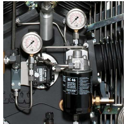
Oil pressure gauge and oil distributor block gauge
